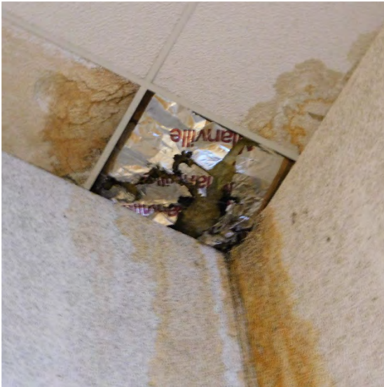
Water damage in the southwest corner of the gymnasium roof
