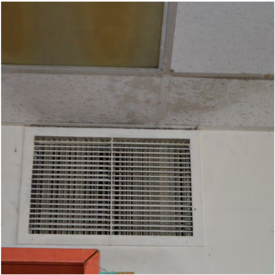
Vents clogged with debris.
