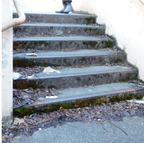
Stair risers and landing chipped, detection strip damaged.
