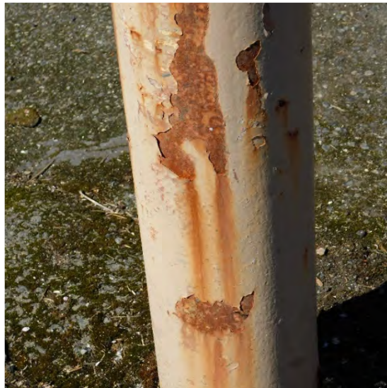
Canopy supports rusted
