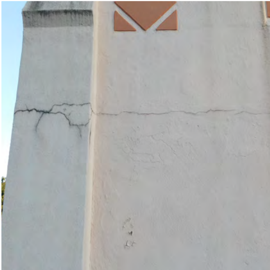
Cracks at wall
