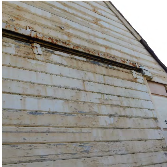
Siding boards damaged, paint peeling
