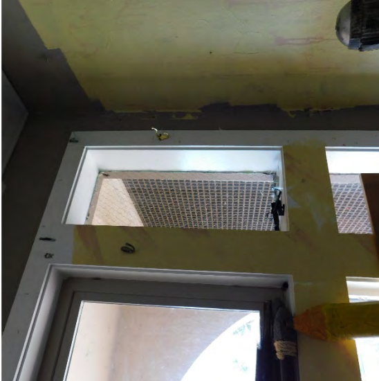
Glazing not code compliant. Damaged window frames
