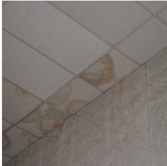
Water damage at ceiling
