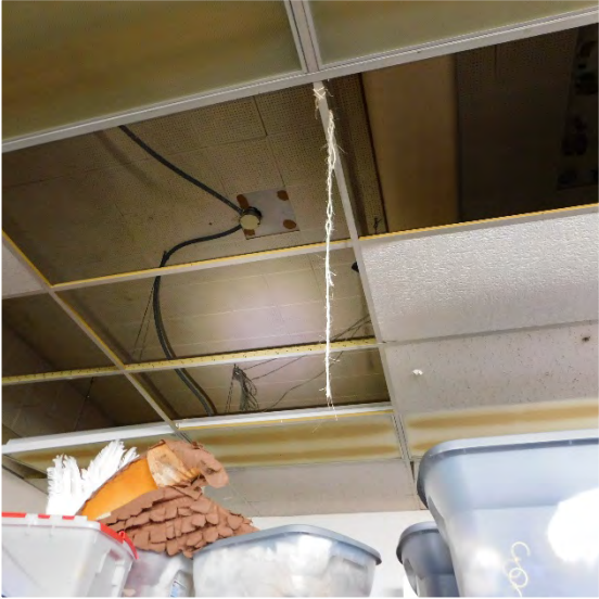
Missing ceiling tiles and lighting
