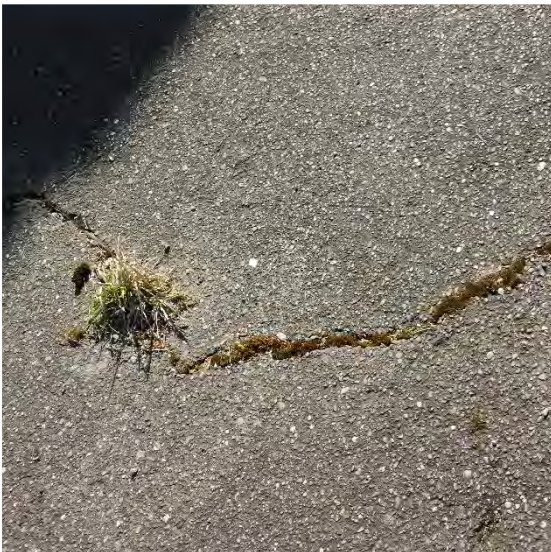
Asphalt pavement cracks
