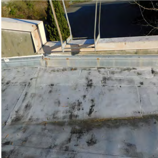
Roof ladder from adjacent roof. Metal coping seperating from the concrete parapet.
