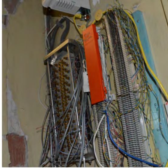
Panel with abandoned wires, not operational
