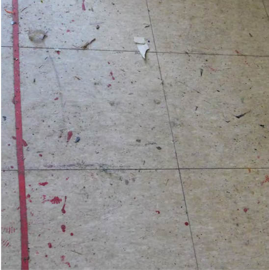
Vinyl tile stained, damaged throughout
