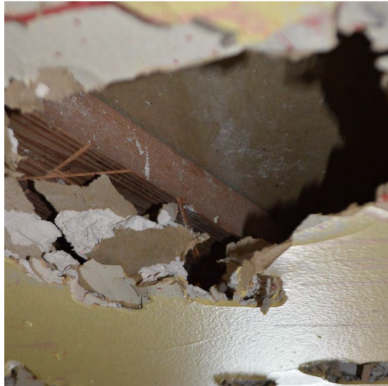
Damaged and punctured walls
