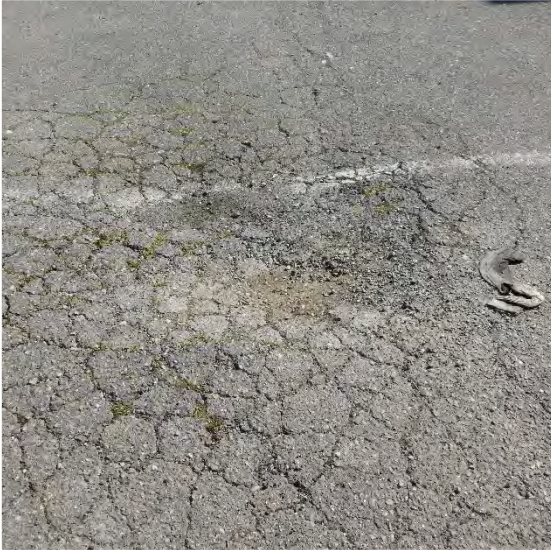
Asphalt pavement cracks and depressions
