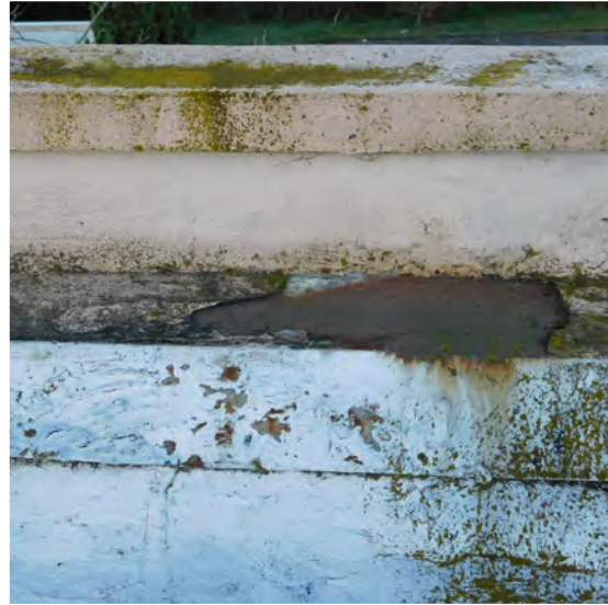
Parapet flashing rusted, roofing membrane punctured, coping cap damage with mildew
