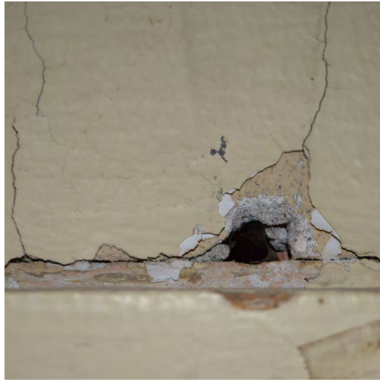
Damaged walls with punctures throughout
