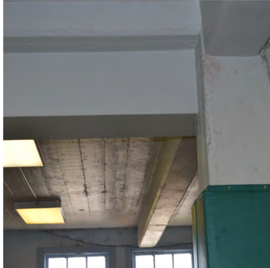
Ceilings no insulation, damaged columns
