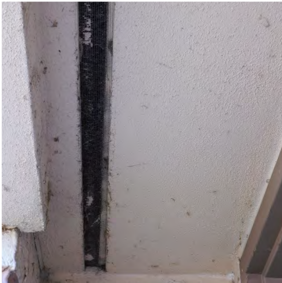
Soffit venting corroded, blocked with debris
