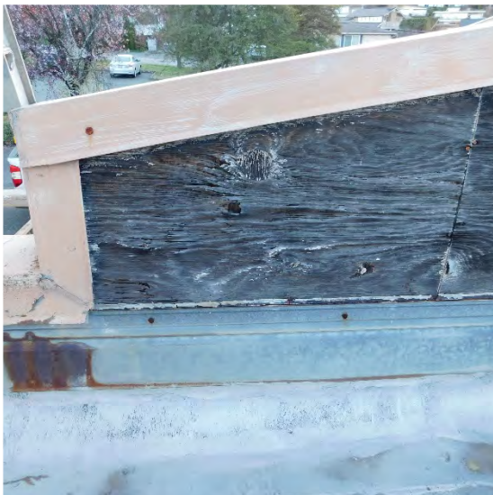
Damaged and wood rot parapet at the lower gym roof
