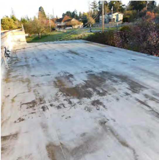
View from upper roof on to lower roof. Very minimal slope and roof system aging
