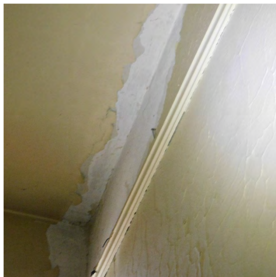
Peeling paint at corners
