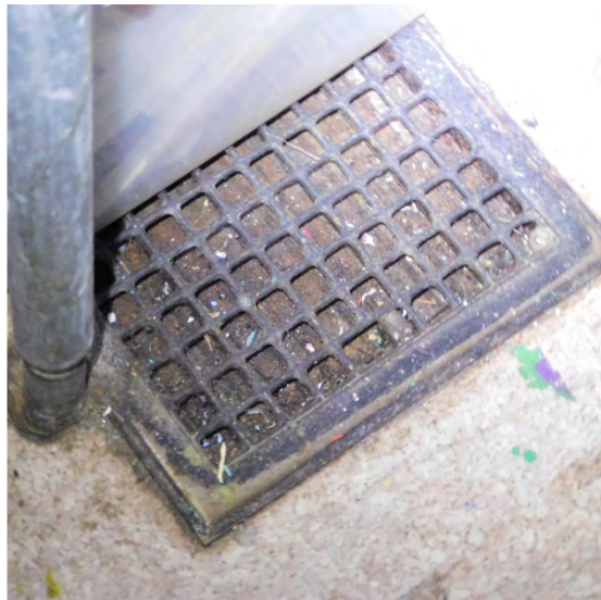
Floor drain blocked by debris, does not appear to be operational
