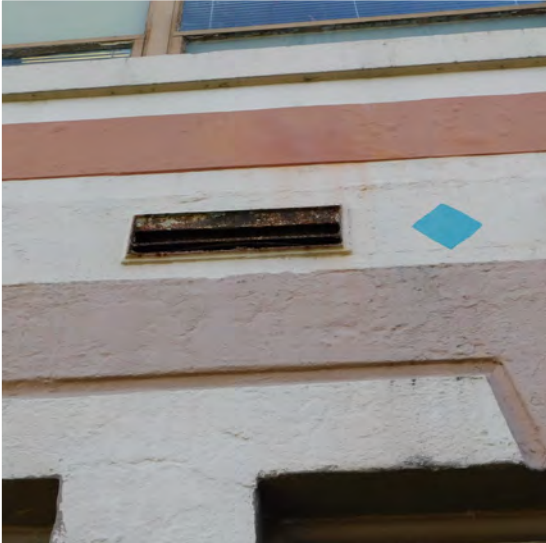
Missing windows, rusted vent shroud
