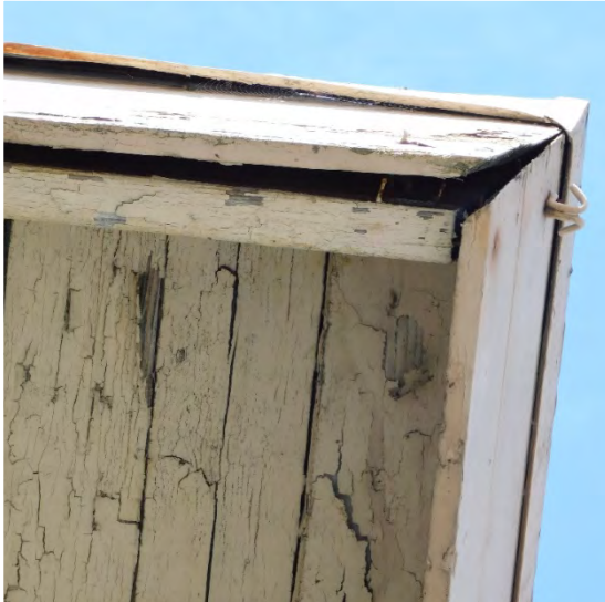
Fascia board and joist connection detachment
