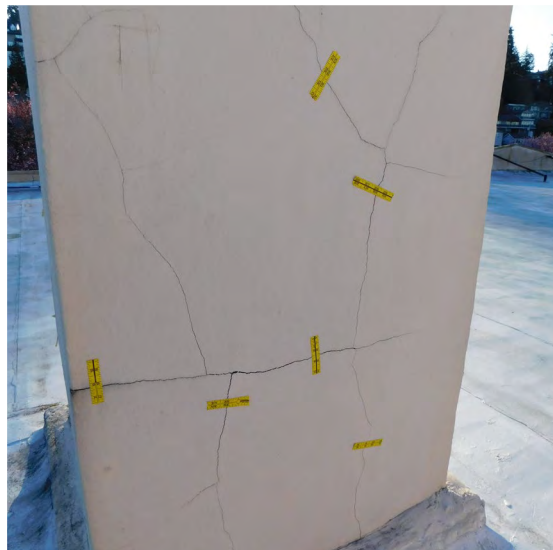
Cracks in the vertical chimney
