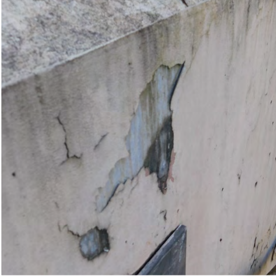
Paint peeling, egress lighting non operational
