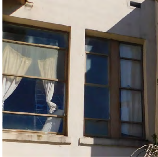
Damage at frames, mildew at window sills
