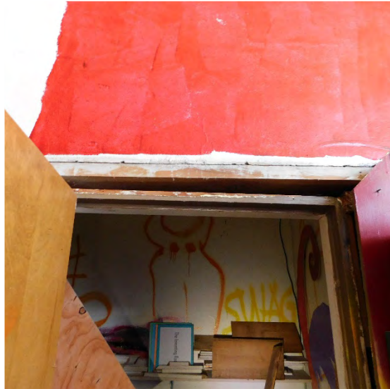
Door frame separated from wall and unoperable. Frame damaged
