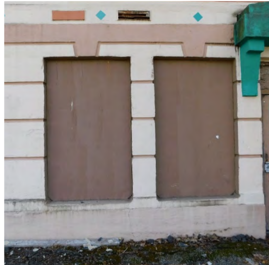
Missing windows, covered with plywood.
