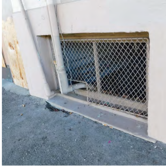
Rusted louvers, penetrations through rated assembly
