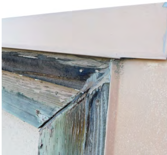
Fascia boards moisture damage
