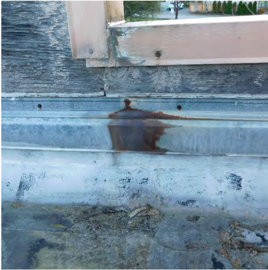
Rusted flashing cap
