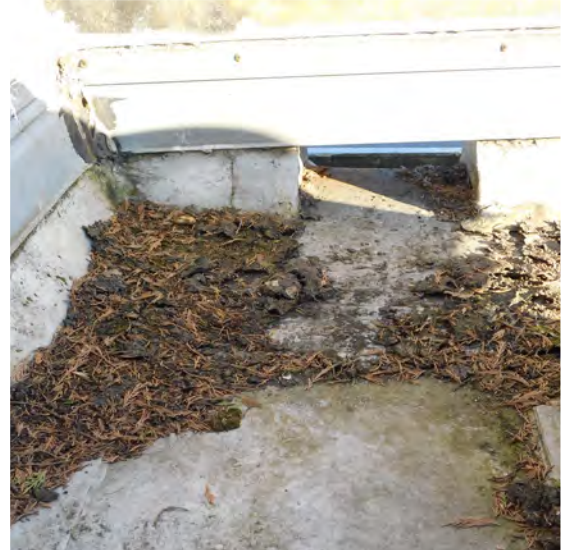
Debris at intervals at roof that block the sloped drainage flow
