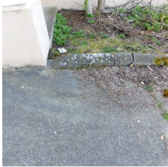
Cracks and damage
