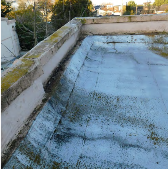
Coping cap damage, mildew throughout.
