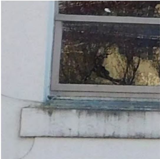
Window sill mildew
