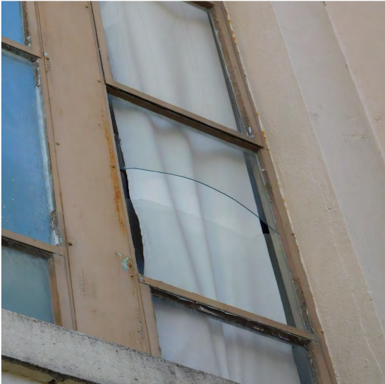
Broken window, rusted window frame
