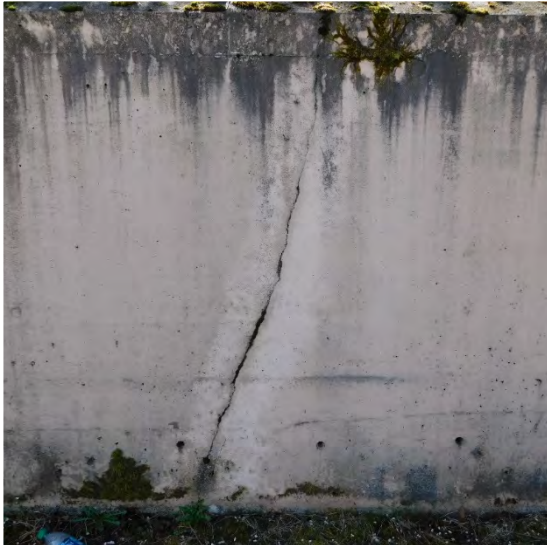
Cracks, decay, damage.
