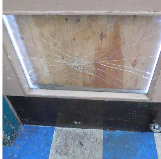
Broken glass in door frames
