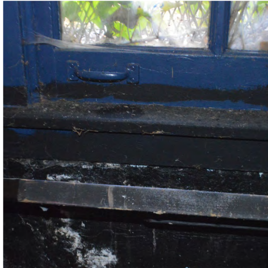
Window framed damaged, not operable
