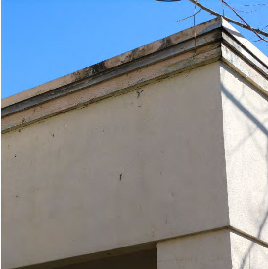
Cornice boards rotted
