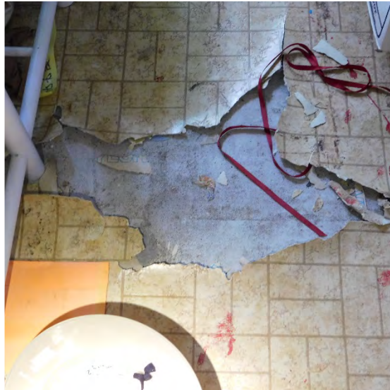
Sheet vinyl floor damaged and missing
