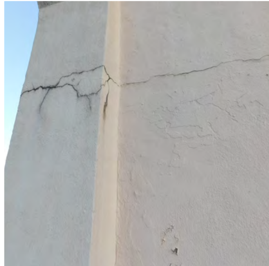
Paint peeling near cracks.
