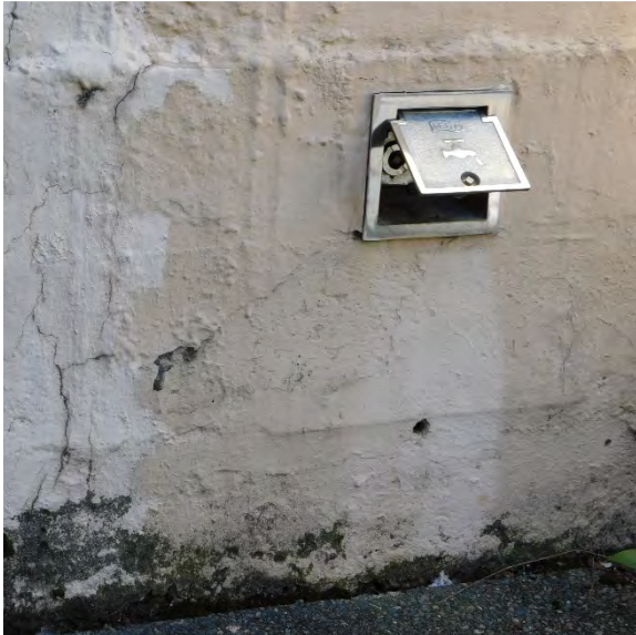
Cracks and substantial mildew
