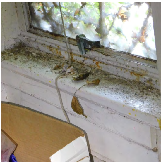
Frames rusted, not operational, single pane glass
