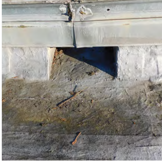
Damaged metal coping. Roof membrane compromised
