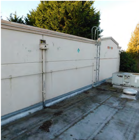
Roof drains from upper roof onto lower with no slope or diversion.
