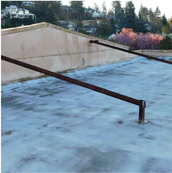
Parapet support bracing rusted
