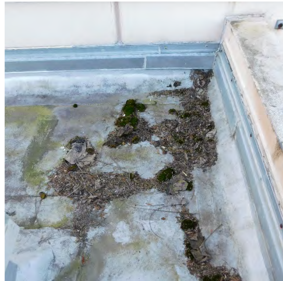
Built-up debris that interferes with drainage pattern. Damage in roof membrane.
