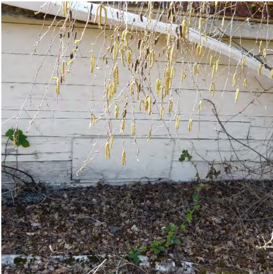
Missing siding boards and vents
