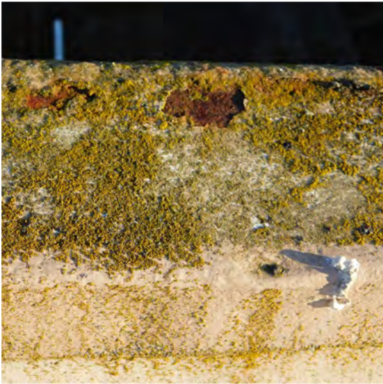
Rusted coping cap, typical at perimeter
