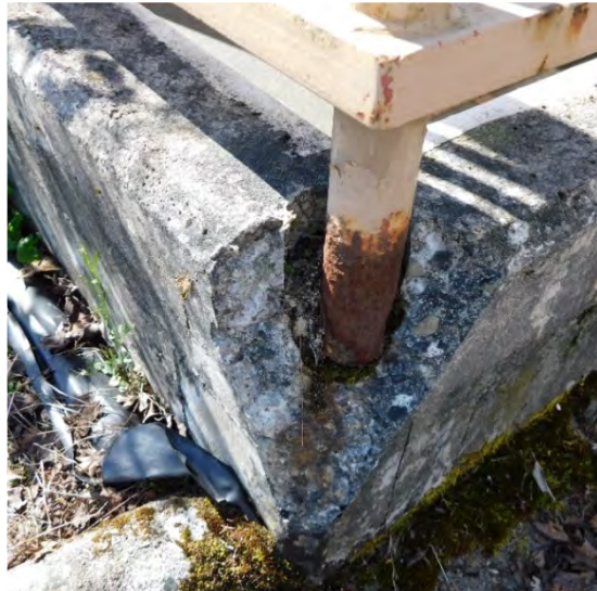
Handrail support rusted, damaged concrete.
