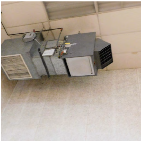
Mechanical unit not seismically braced
