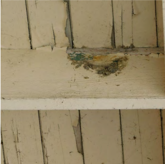
Boards water damage
