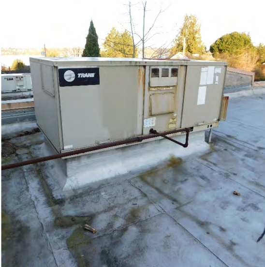
Mechanical Unit lines rusted, unit itself lacks regular service information.
