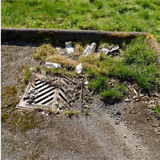
Catch basin drainage blockage
