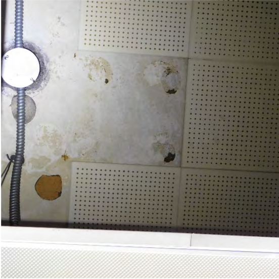
Hard-lid ceiling tiles separating detached from structure. Damage in concrete ceiling
