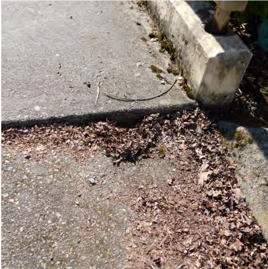
Transition from parking lot to stair landing grade difference.
