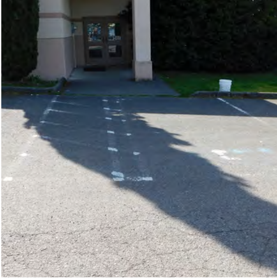
Accessible parking not code compliant
