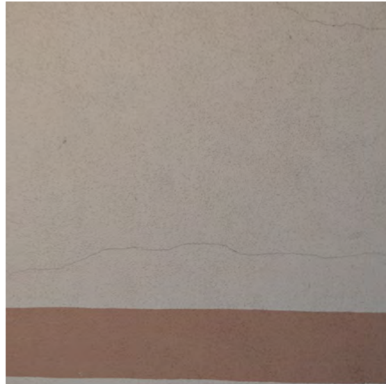
Cracks in stucco finish
