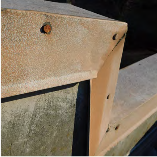
Rusted metal coping cap and fasteners
