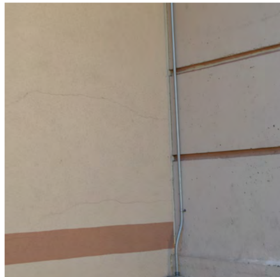
Buildings attached, no expansion joint
