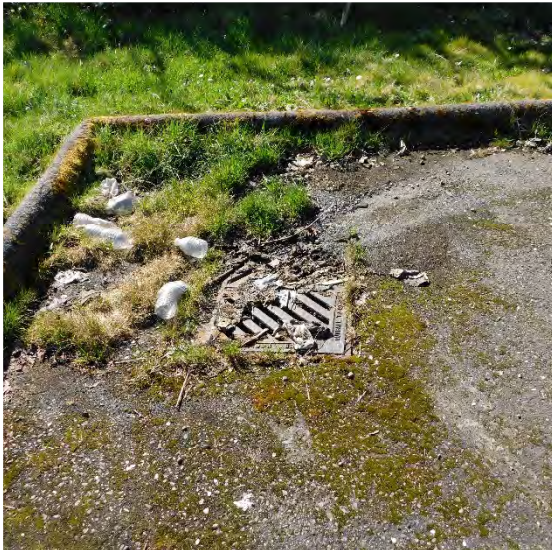
Catch basin drainage blockage
