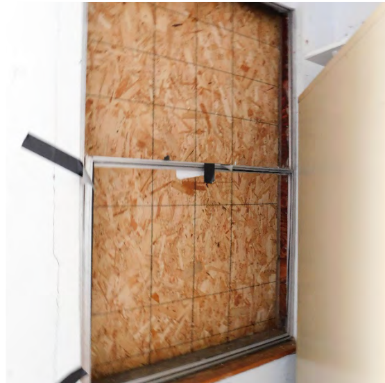
Window glass missing, frame perimeter damaged and not operational
