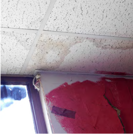
Water damage at ceiling
