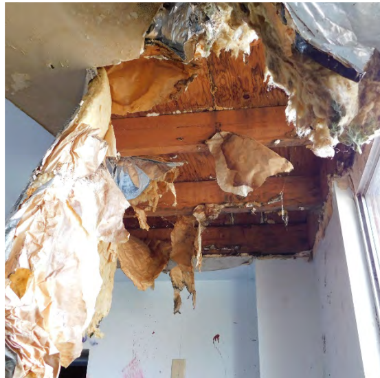
Water damage at ceiling. Exposed structure
