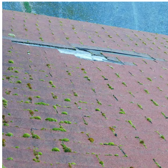
Missing roof shingles
