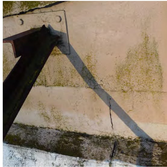
Support bracing attachment rusted with attachment unstable since attached to sheet metal
