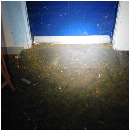
Floor transitions added to access rooms. Slope of material damaged and chipped.
