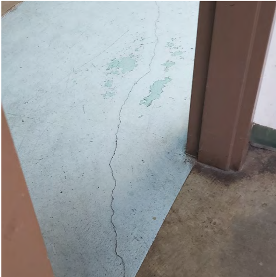
Cracks in concrete floor
