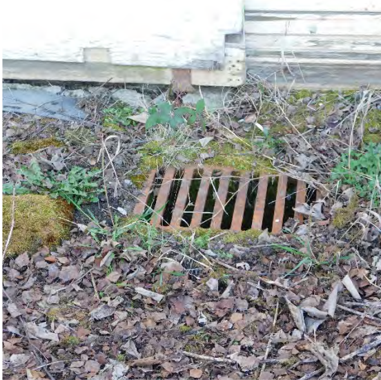
Catch basin drainage blockage
