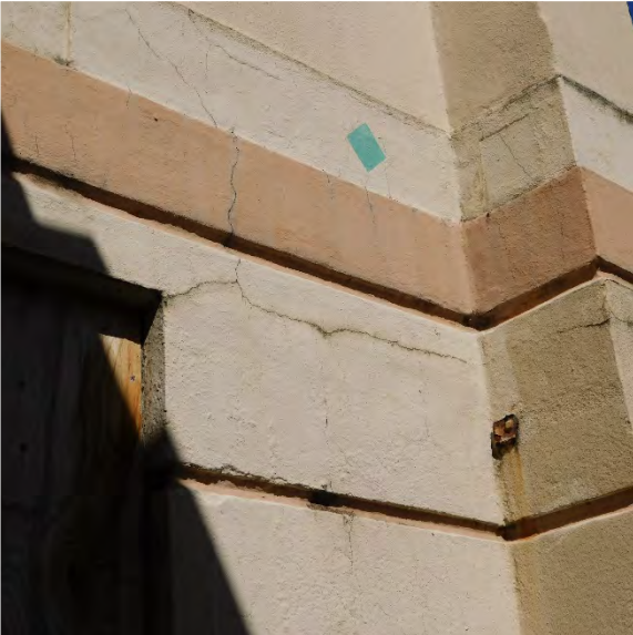
Concrete cracks and rust
