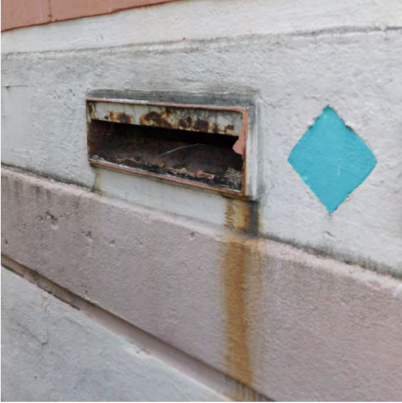
Rusted vent shrouds
