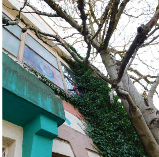
Concrete roof and brackets covered in mildew
