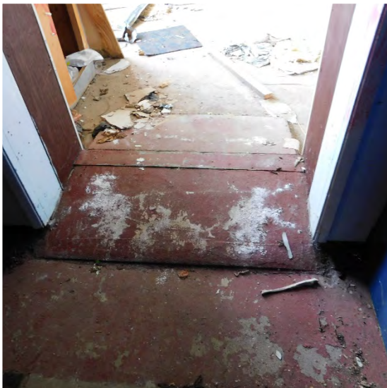
Floor transitions added to access rooms. Slope of material damaged and chipped.
