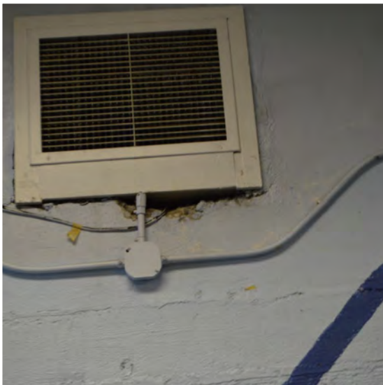
Ventilation penetrations cracked, not in operation
