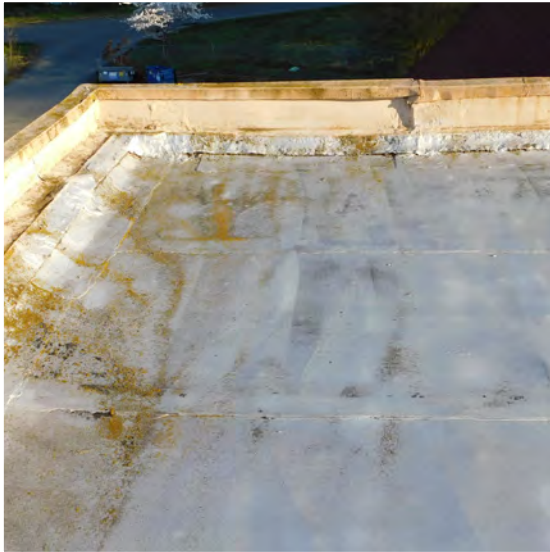
Roof lapping seams peeling
