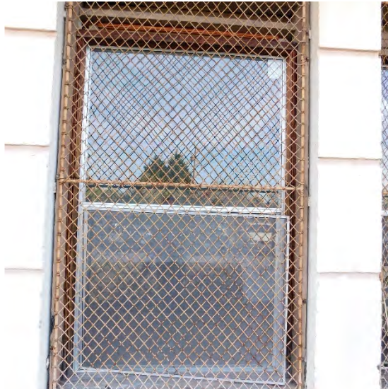
Windows failing, mesh rusted
