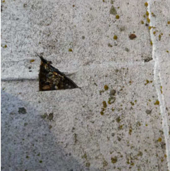
Punctures through the roof membrane
