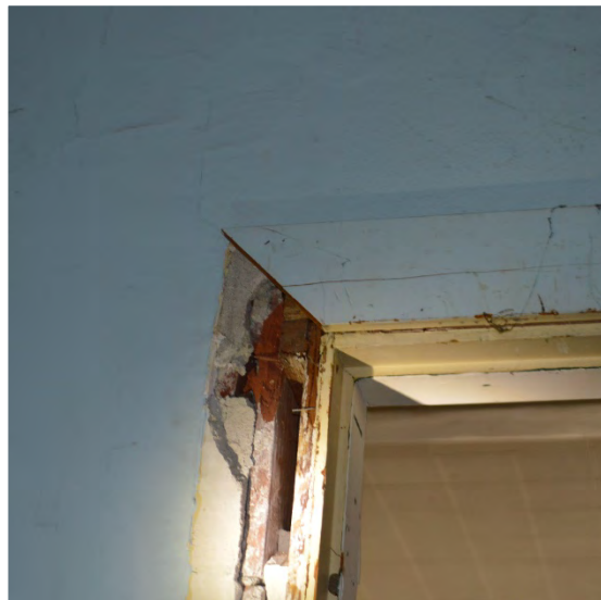
Frames missing, damaged
