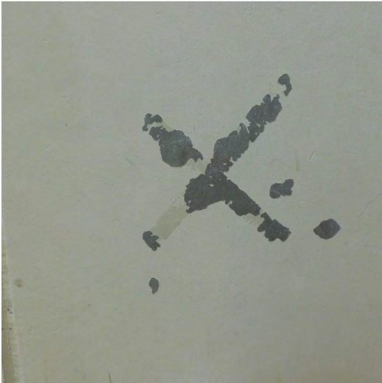
Paint missing, damage in parts of wall.
