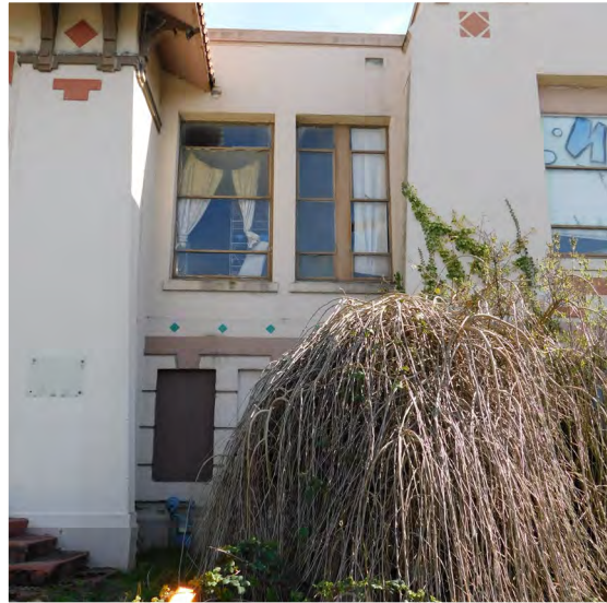
Trees pruning lack of maintenance
