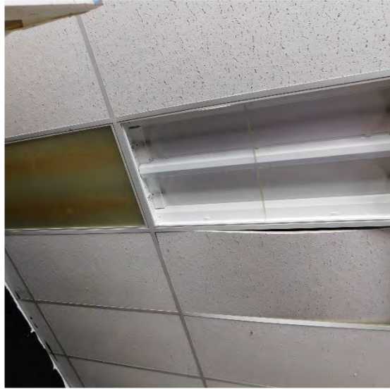
Missing light fixtures, tiles not set in place. No seismic bracing of the ceiling.
