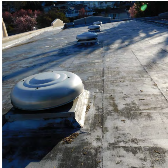
Roof membrane seams separating, peeling
