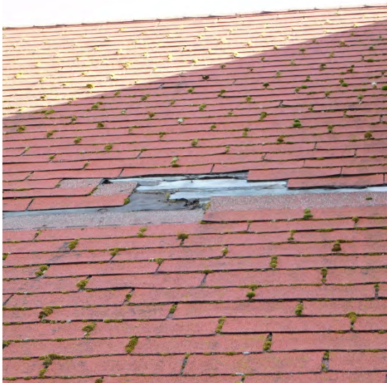
Missing roof shingles which compromises roof integrity
