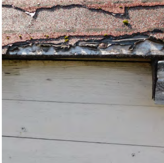
Roof damage, missing fascia boards
