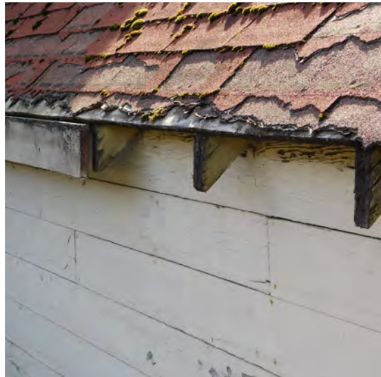
Missing fascia boards and gutters
