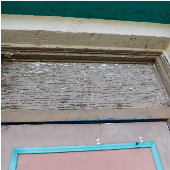
Door wood frame damaged, transom glass missing replaced with wood.
