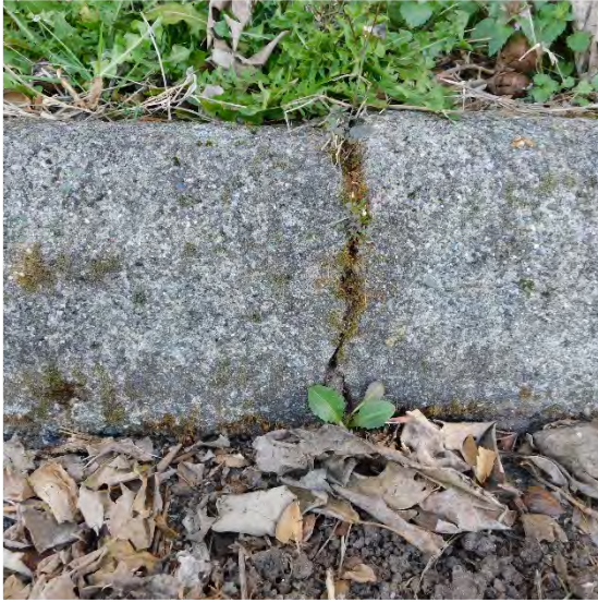
Cracks and damage
