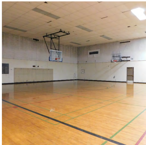
Light fixtures not in operation
