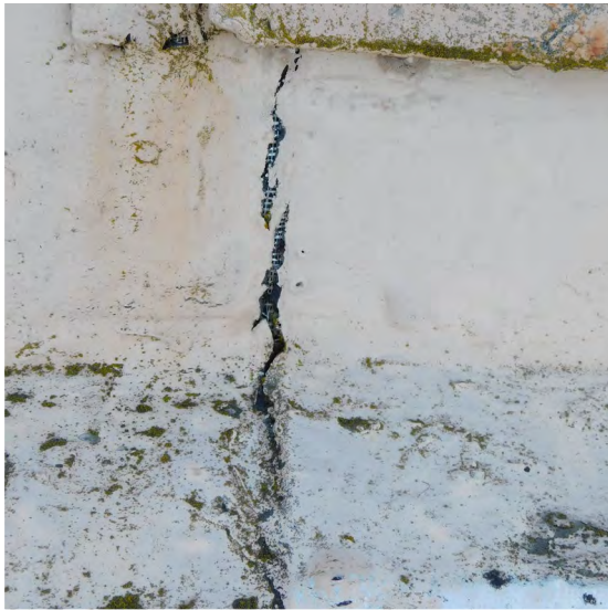
Roofing material cracking
