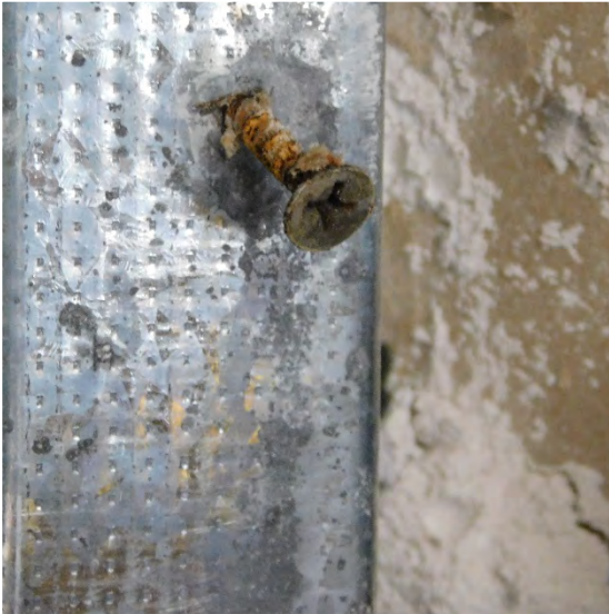
Exposed nails, rusted, and framing. Missing drywall finish
