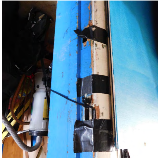
Wall interface with door jams attached with tape and other methods
