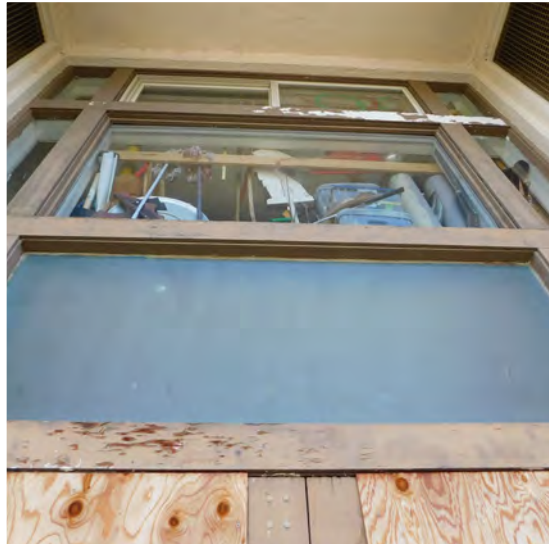
Transom glass missing, frames damaged.
