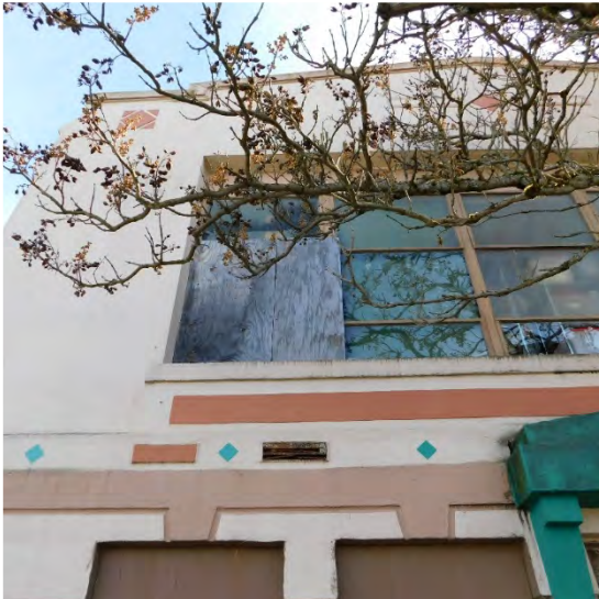
Missing windows, rusted vent shroud
