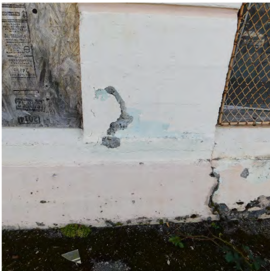
Cracks in concrete at west elevation
