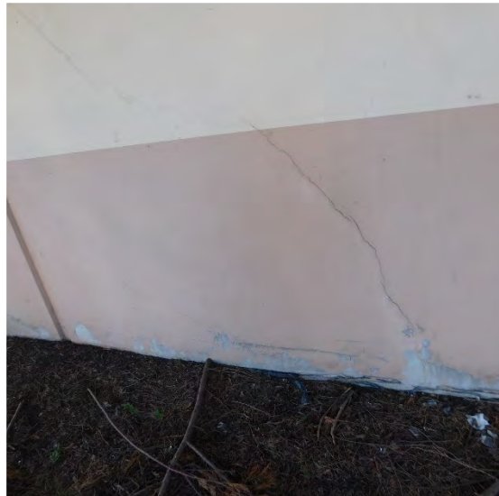
Cracked concrete wall
