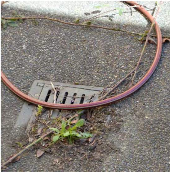
Catch basin blocked with debris at entry of gymnasium
