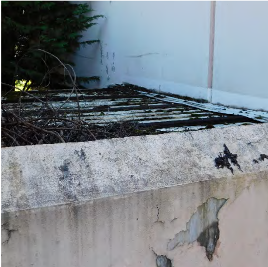
Cracks, paint chipping
