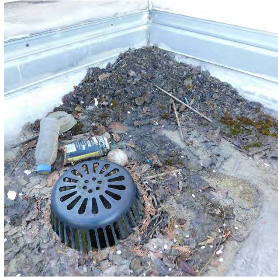
Downspouts compromised due to debris, mildew buildup
