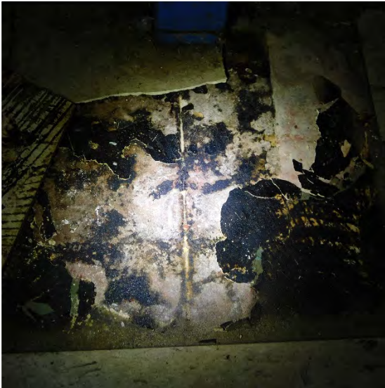
Vinyl square tiles missing, mastic exposed.
