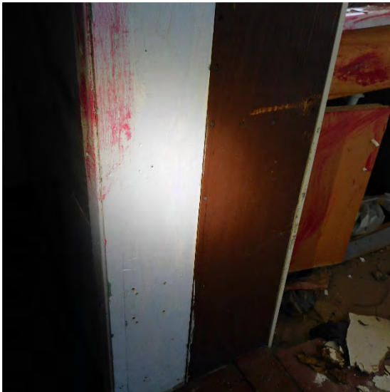
Wall finish at door jambs damaged
