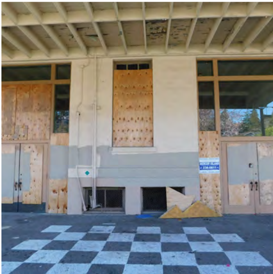
Missing glazing, sindows and frames
