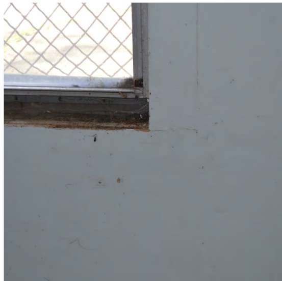
Missing window sills, framing exposed
