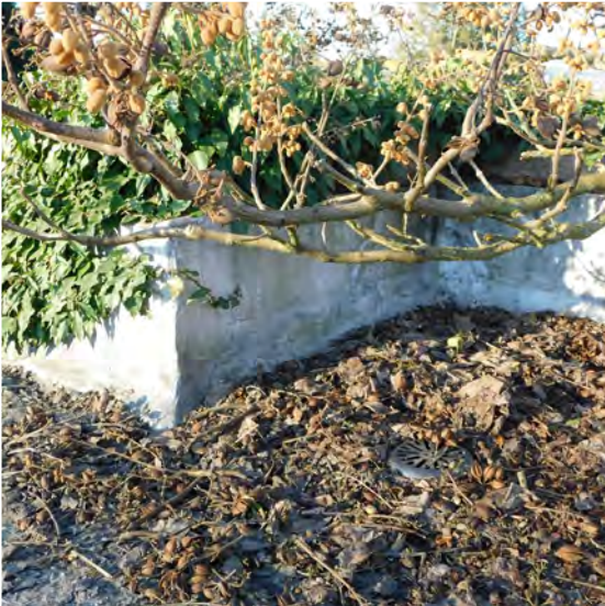
Downspout blocked with debris
