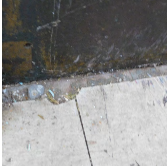
Missing transition strips to bridge different materials
