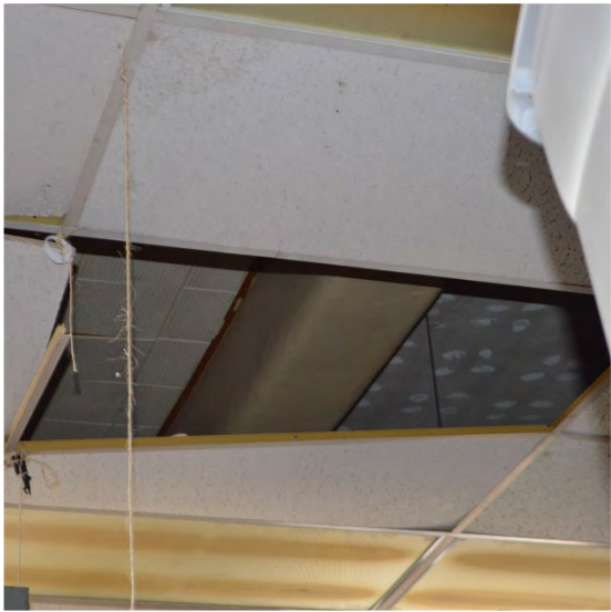
Ceiling within a ceiling. Tiles detaching and going through the ACT ceiling.
