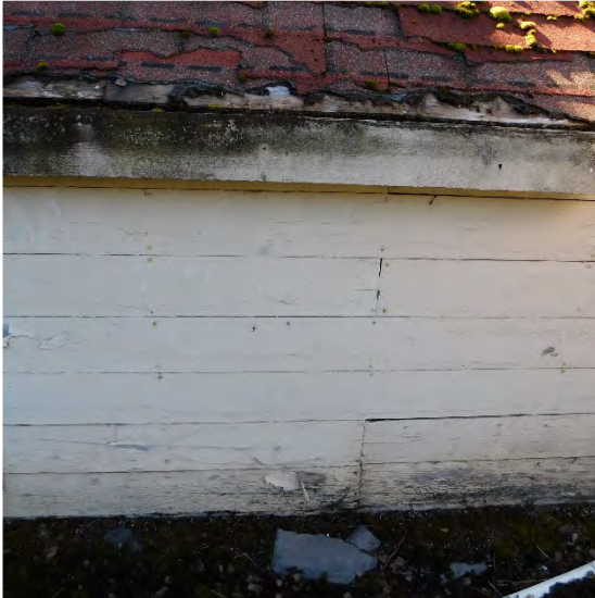
Wood rot and mildew throughout
