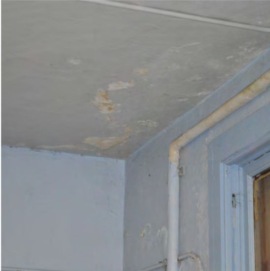
Paint peeling, missing window.
