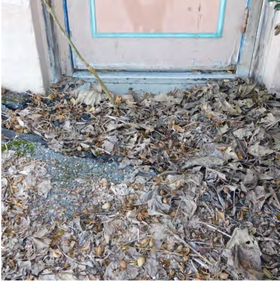
Asphalt paving damaged. Door threshold, slope, and threshold insufficient.
