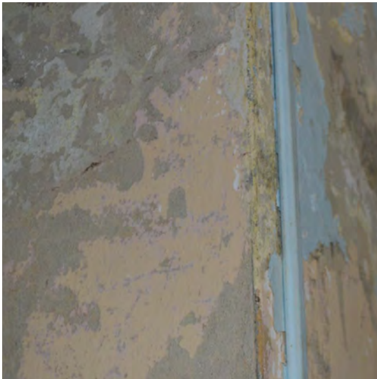
Damaged walls with no interior finish
