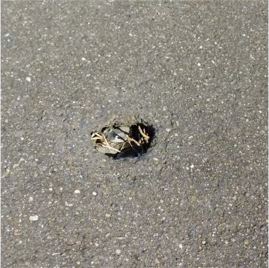
Depressions in asphalt
