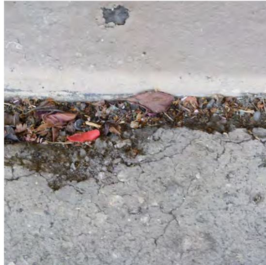
Damage at buiding entry interface to asphalt
