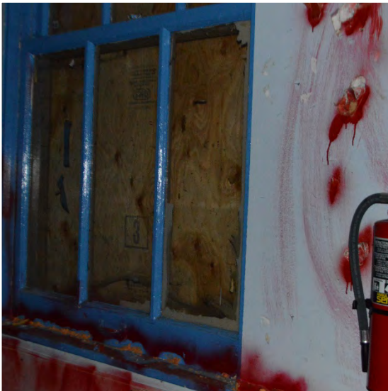
Missing glass, frames damaged
