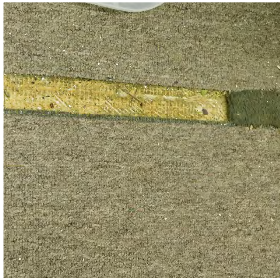
Transition strips missing
