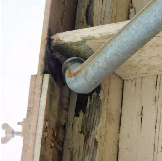
Water damage at roof drain connection
