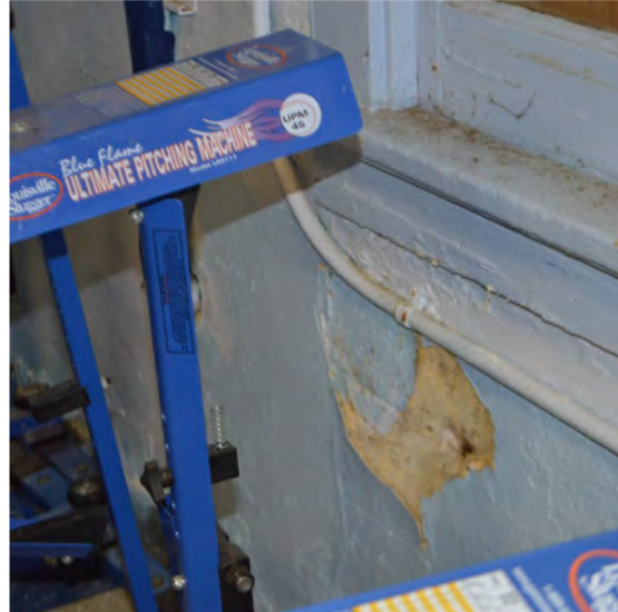
Damage in walls. Concrete walls only no interior insulation or walls
