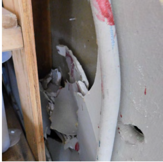
Drywall finish damaged, exposed framing
