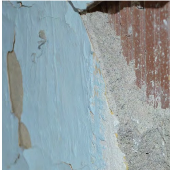
Exposed and damaged walls throughout
