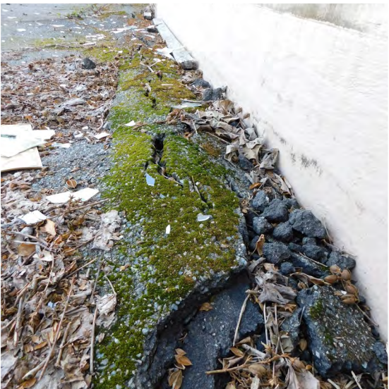
Asphalt pavement damage at building
