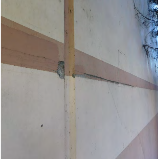
Cracks in concrete wall
