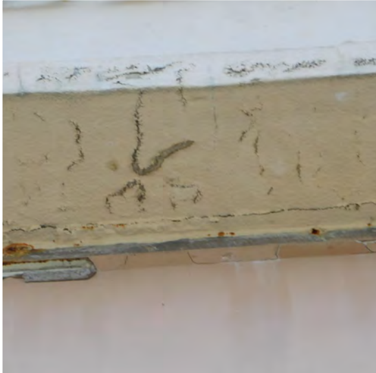
Cracks in concrete at exterior window soffit.
