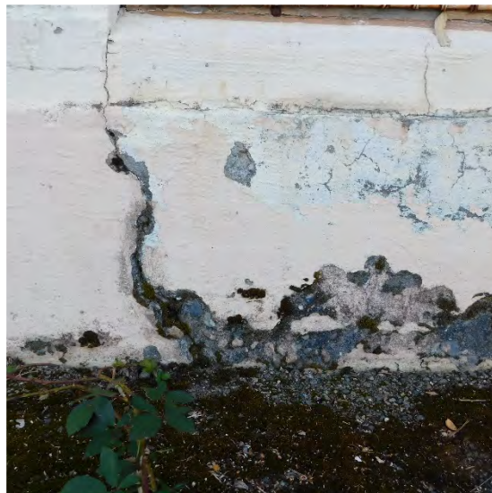
Cracks in concrete at west elevation
