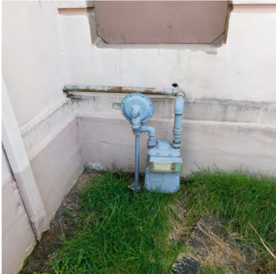
Utility rusted penetrations in concrete
