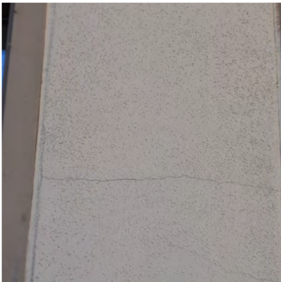
Cracks in stucco finish
