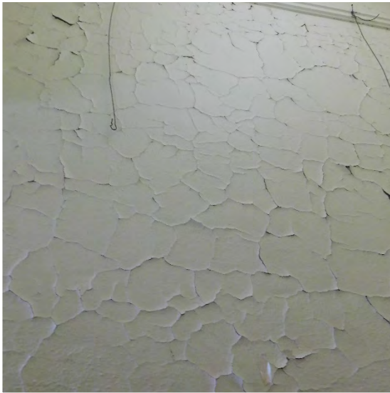
Paint peeling throughout at all masonry walls
