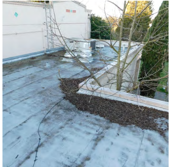
Roof blocked by debris which interferes with roof drainage patterns and flow
