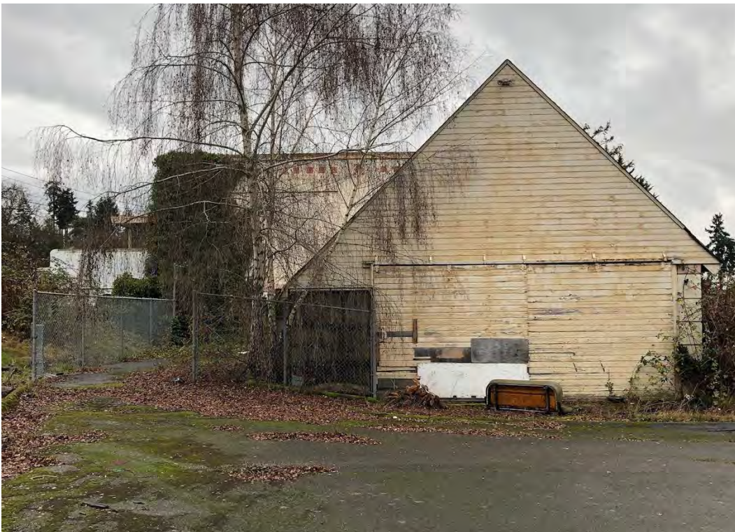
Looking south at the north end of the playshed and north end of original school building partially visible beyond.
