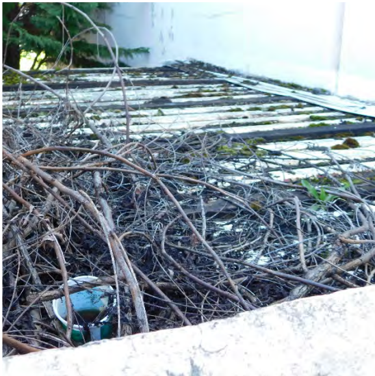
Metal roof at outside storage at building damaged, blocked with debris. No visible drainage
