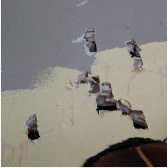
Damaged walls with punctures throughout.
