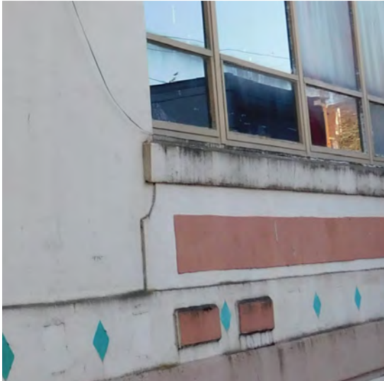
Mildew at exterior wall
