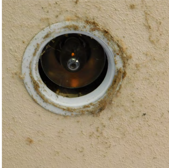
Corrosion at soffit light fixtures
