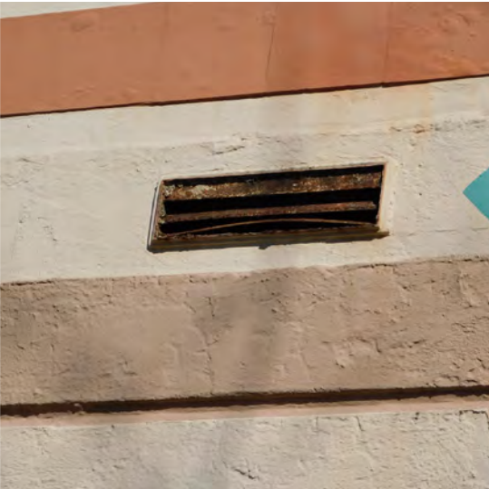
Rusted vent shroud
