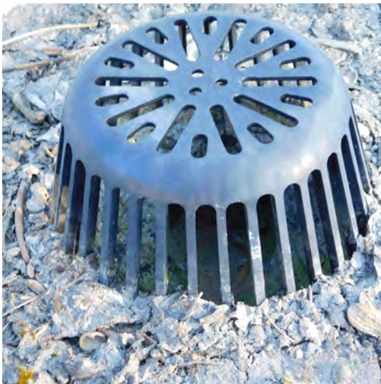
Downspout blocked. If water can not get out then will pond on roof
