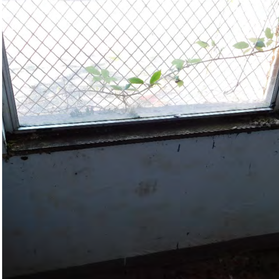
Window frame damaged, condensation at perimeter
