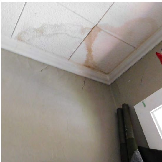
Water damage at ceiling
