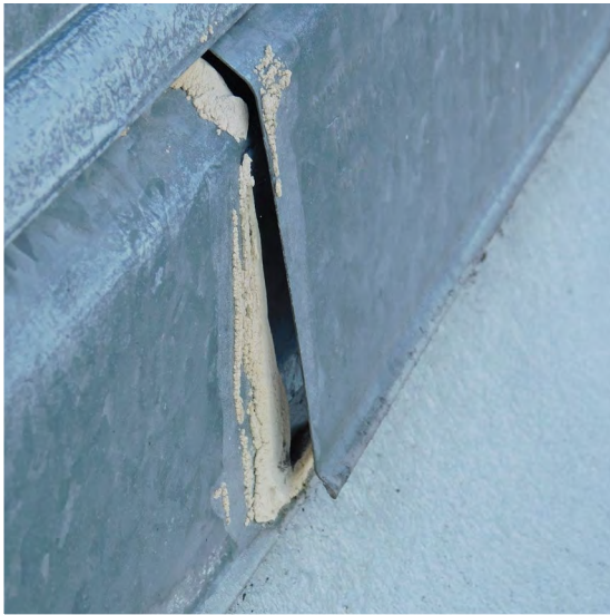
Parapet coping cap damaged
