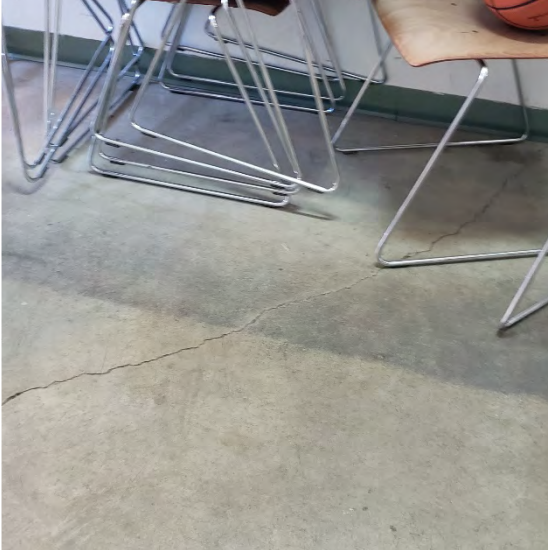
Cracks in concrete floor
