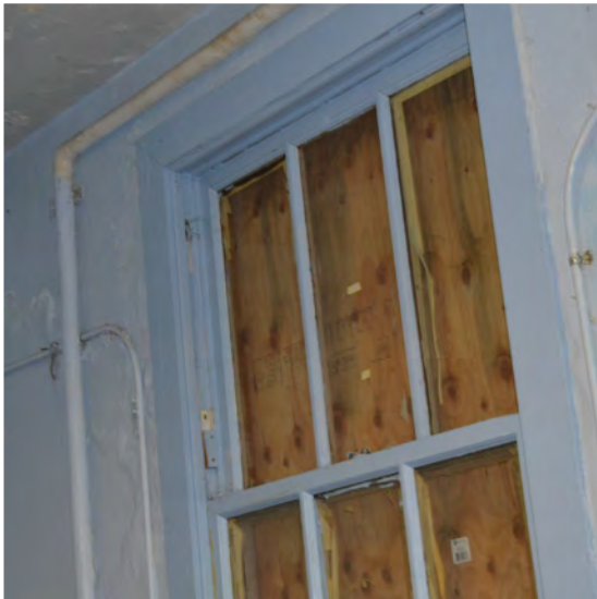
Window missing glass
